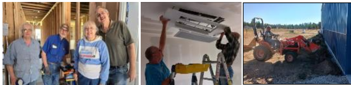
Above Photos: Left: Bill & LaVonne made 3 trips to help with electrical, generator, painting and clean-up at our pole barn! Middle: Rich and Bill installed 4 Mr Cool heating/cooling computerized ceiling heads. Right: Rich placed metal over the wood foundation skirting before our 86-yr.-old neighbor, Joe, used his tractor to scoop excavated dirt and dump it against 3 sides of our pole barn to meet an occupancy elevation water run-off requirement. He and another friend helped mow down weeds also.
