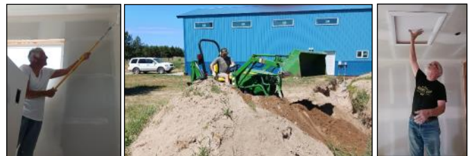
Above Photos: Left: Wendy helped paint. Middle: Pastor Justin refilled a trench in June, burying plumbing pipes 4-ft. deep from the utility room in building to the well head. Right: Kim helped install the attic hatch, 2 fire doors and, and more plumbing. We are so grateful for volunteer help God provided just when we needed it!
